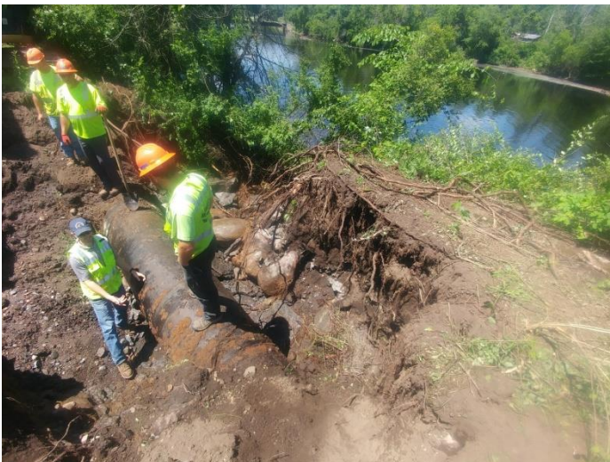
Inspecting leaking section of 36" pipe 10' long crack along bottom.
