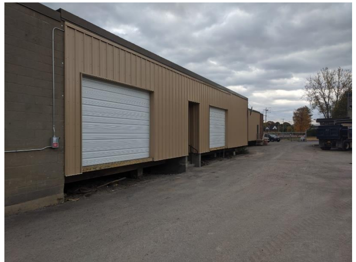
Work was undertaken to eliminate rain and snow intrusion, and to keep birds out of interior.
