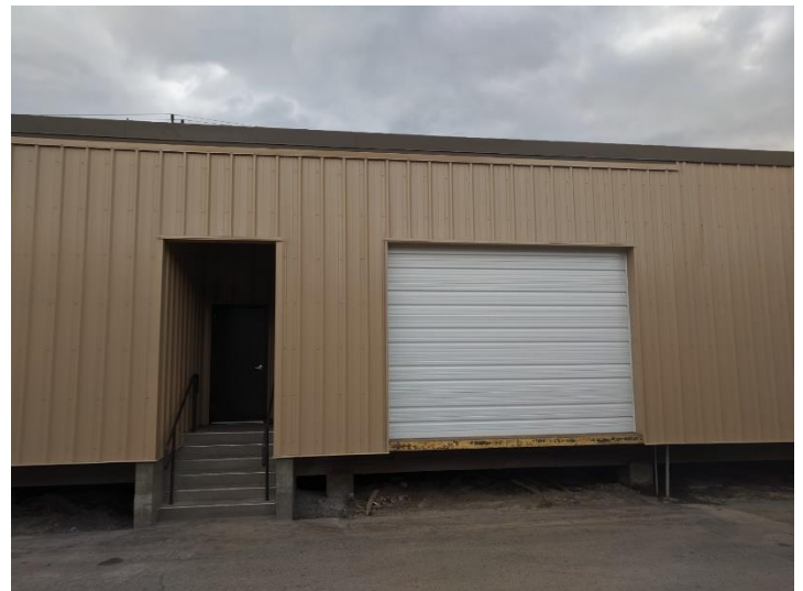
Work was undertaken to eliminate rain and snow intrusion, and to keep birds out of interior.
