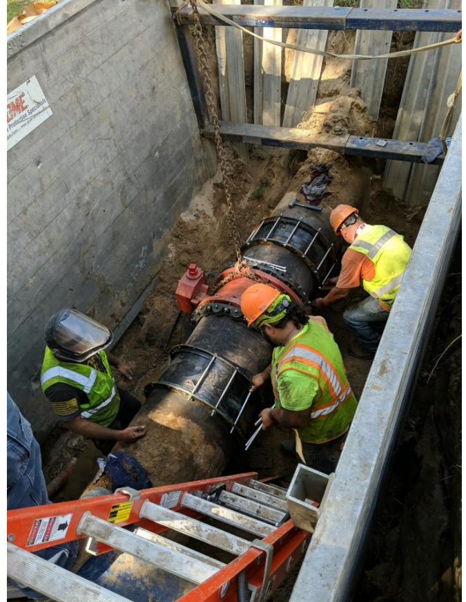
New 24" Butterfly Valve Installed. New Couplings Used to Connect to Existing Mains.
