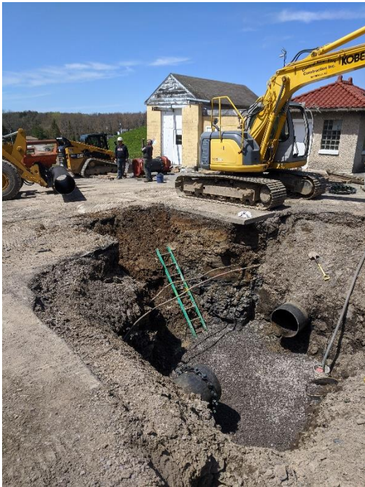
Excavation for connection to existing 24" water main. 100 ± year old main was found in very good condition.
