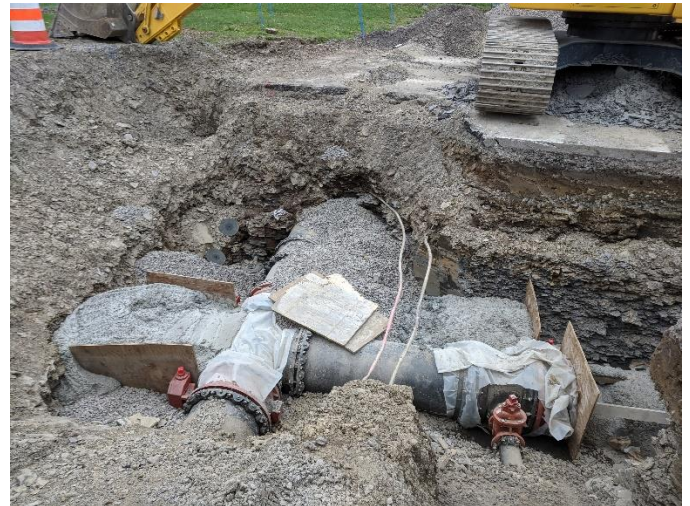
Connections installed with two (2) new 24" isolation valves. Concrete thrust blocks poured to include stabilize pipe against pressure induced movement.
