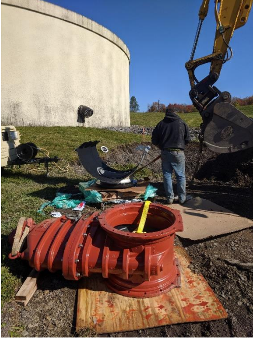
Preparation to mount Tapping Sleeve & Valve on existing 4" main outlet from Cavanaugh Road Water Tank.
