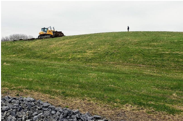
First earthwork cut into the Reservoir Embankment. All work is being completed by MVWA crews.
